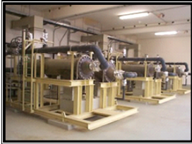
MGPS & Anti-Fouling System
